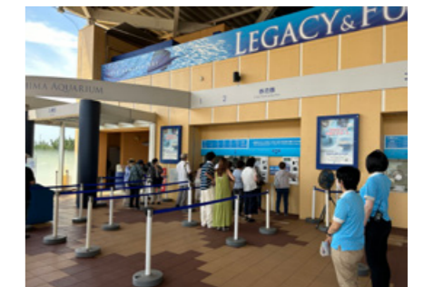
KC-TS30IQ units installed at the ticket counters
